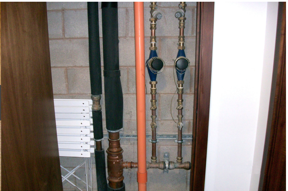
Pipework feeding the apartments installed correctly
